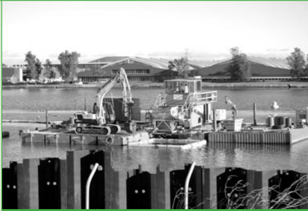
Above: Removal of sediment is performed on a floating barge by an excavator fitted with a "clam-shell" bucket.
