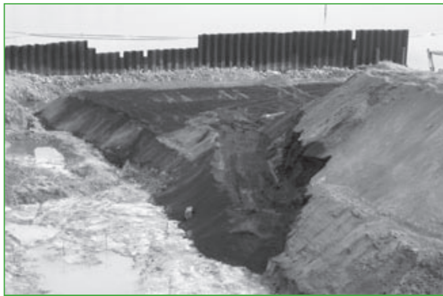
Above: Dark, treated soil is backfilled across a clean and natural, excavated surface
