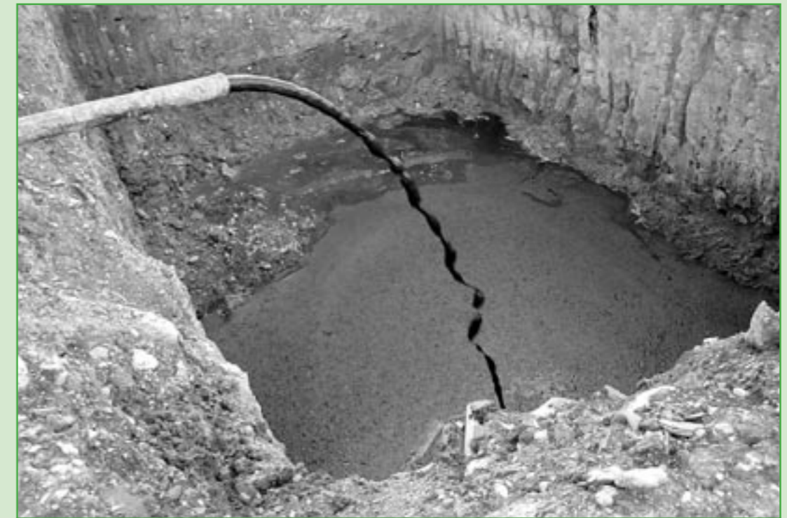
Above: Excavated bay sediment is pumped into pits where it is tested for chemical constituents.
