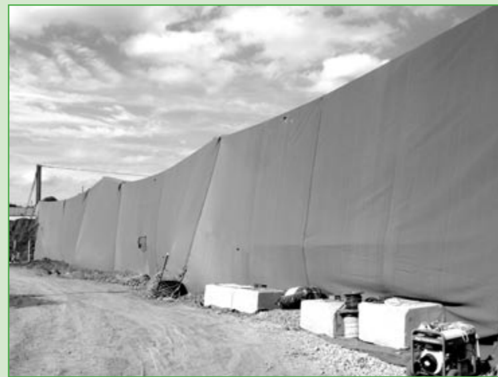
Above: The new odour-control enclosure over the contaminated soil storage cell on the Lednez site.
