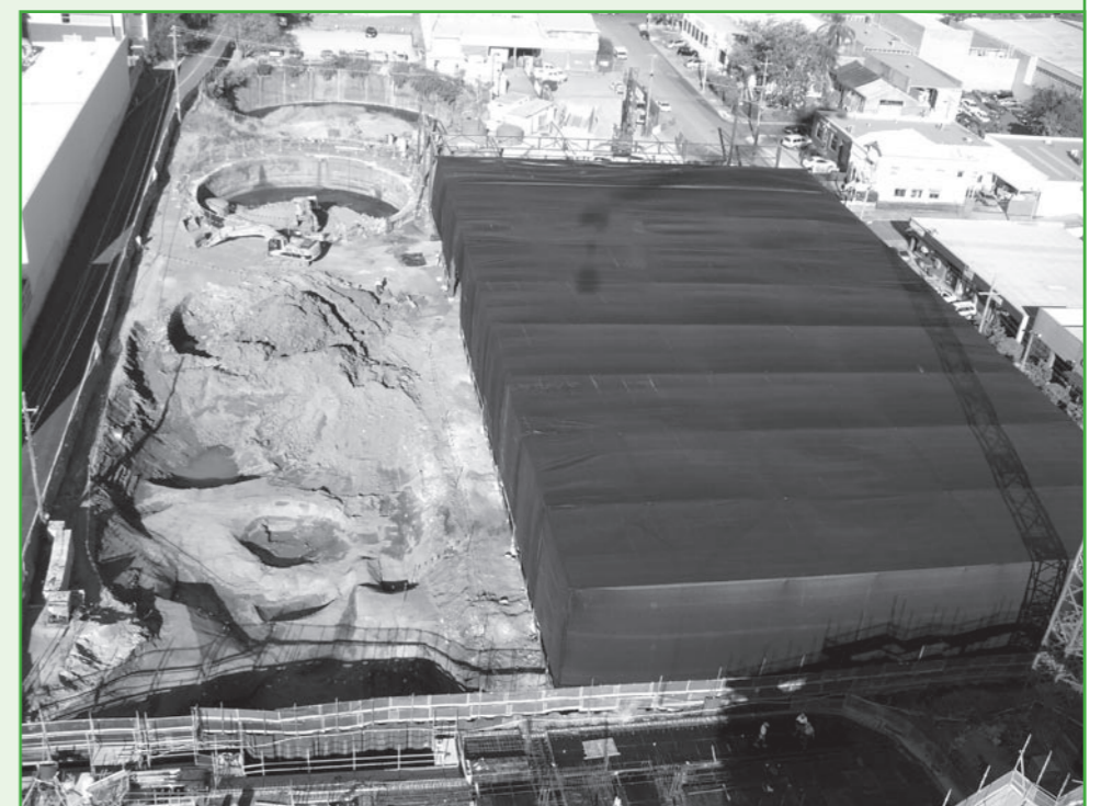
Above: To help minimise odour, a structure similar to the one above will be built over the contaminated soil containment pit on the Lednez site.
